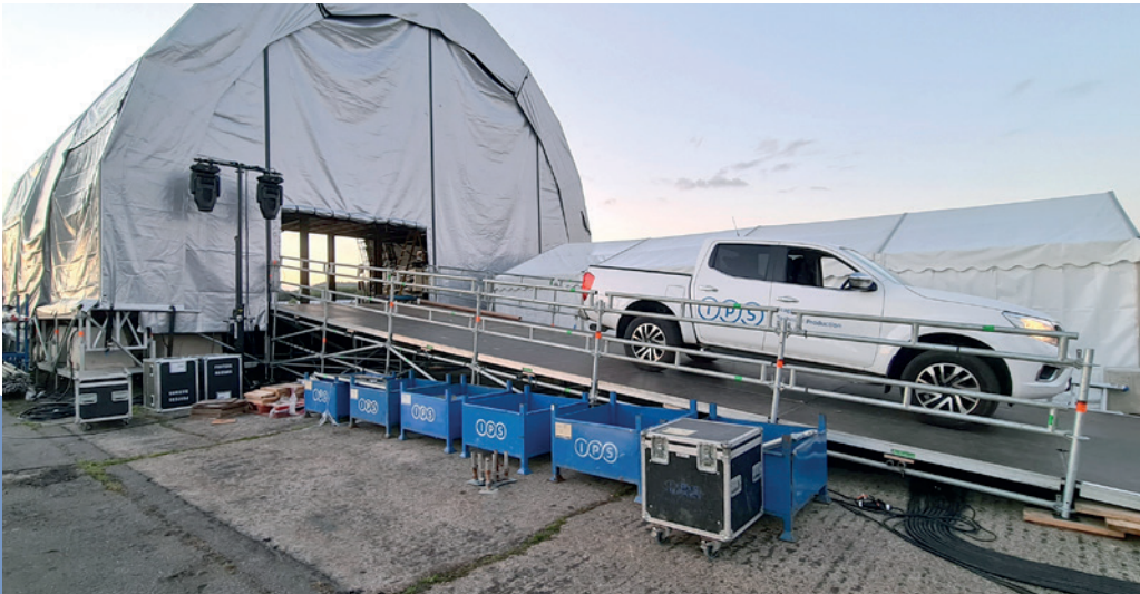
15m Custom vehicle access ramp constructed to rear of Top Gear Structure
