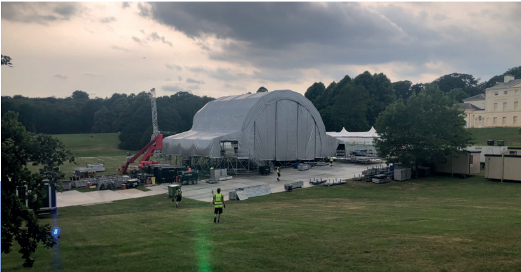
18m Structure during construction on sloping site. Structure shown with additional truss PA towers
